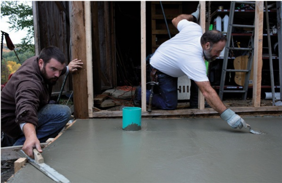
RIGHT: Joe Jones, left, and his father Bruce Jones of Jones Roofing and Masonry in Chelsea, Vermont. smooth fresh concrete poured for the roof of the new root cellar at Fat Rooster Farm. The vent at center is one of two used to regulate airflow and temperature in the cellar.
